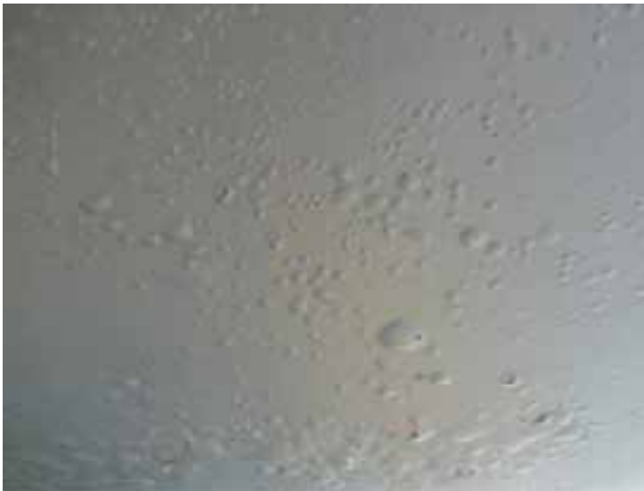
Osmoseschaden in fortgeschrittenem Stadium
